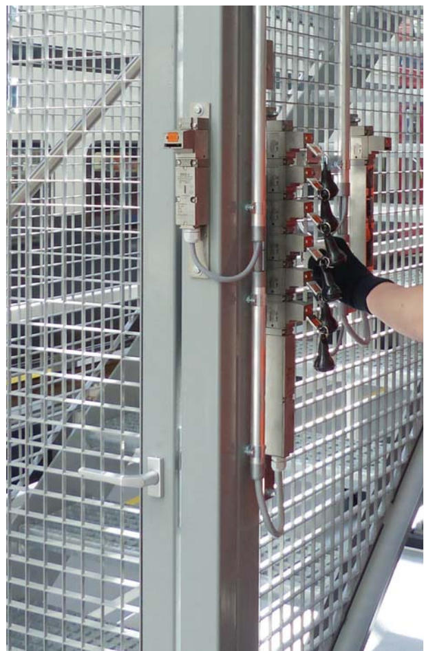
Example of a key changer: The sign on the door also indicates that access to the secured area is only permitted with one key per person
