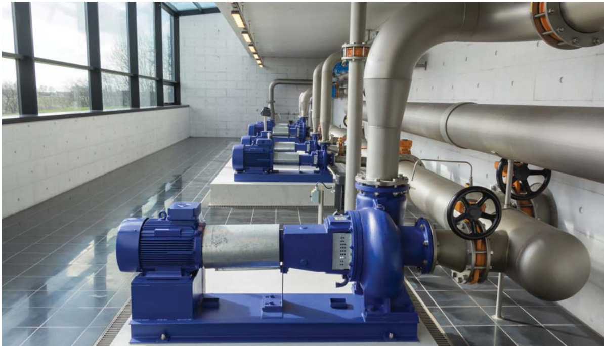
Electrically operated pumps in earthed networks, which are predominantly switched off, cannot be permanently monitored with residual current monitors.
