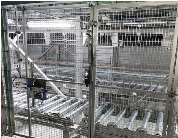
The facilities for the production of deep-frozen vegetables in Reken are largely installed in the refrigerated area.
