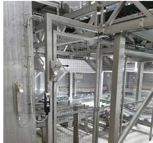
The doors are safeguarded with the SAFEMASTER STS system.
